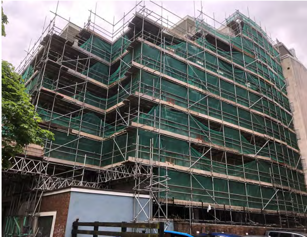
Photograph 3: View of Tŷ Cambria with substation structure, facing south-east from the access road to the north of the site.
