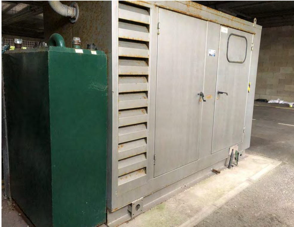
Photograph 5: View of substation outlet and tank located within the existing undercroft parking at the site.
