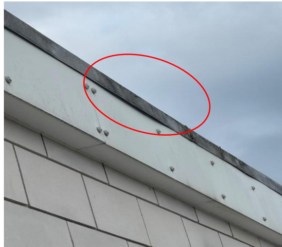
Figure 13 – Potential Roost Feature (PRF 2) of raised lead flashing.
