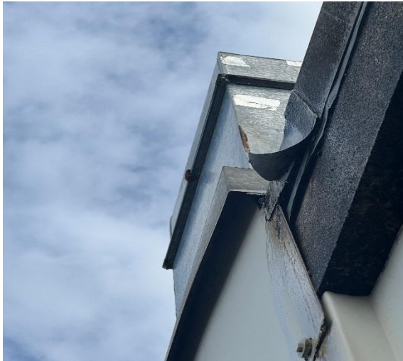
Figure 12 – Potential Roost Feature (PRF 1) raised lead flashing.
