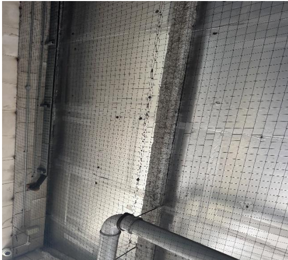
Figure 8 – Example of netting within car park.
