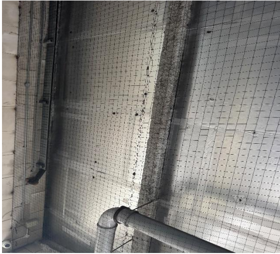
Figure 8 – Example of netting within car park.
