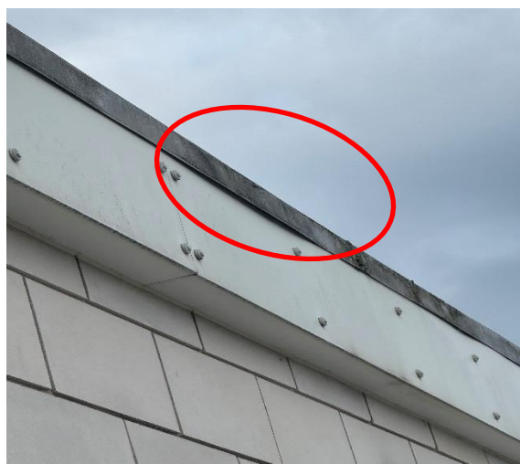
Figure 7 – Example of raised lead flashing.
