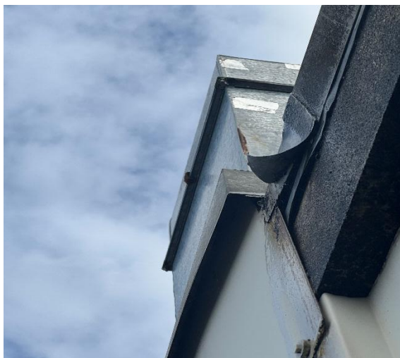
Figure 6 – Example of raised lead flashing.
